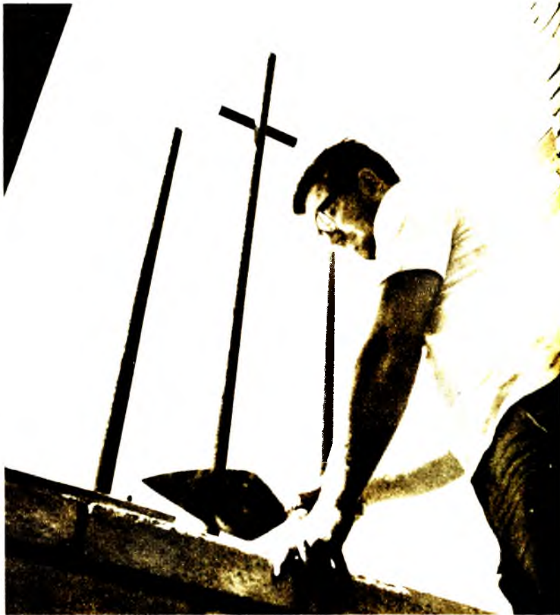
CONSTRUCTION NEAR END—A workman lays another brick to bring the new church building at Redding, California, nearer completion. The building, which will have wall-to-wall carpeting and new appointments, is scheduled to be completed about November 1, according to Pastor Virgil M. Hultcheson.
